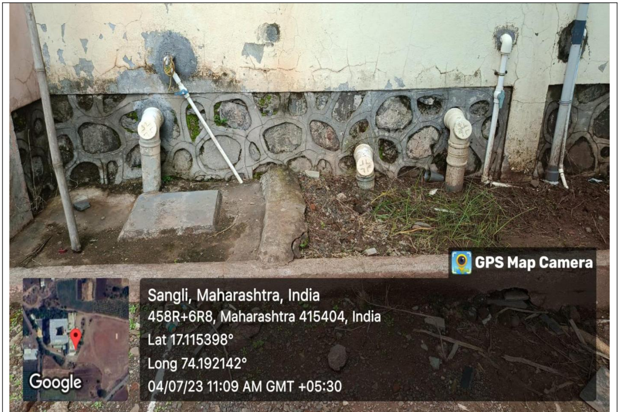
Pipe of Toilets
